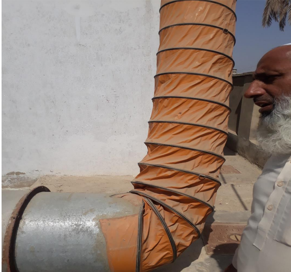
Figure 11: Exhaust duct for solar drying unit.
