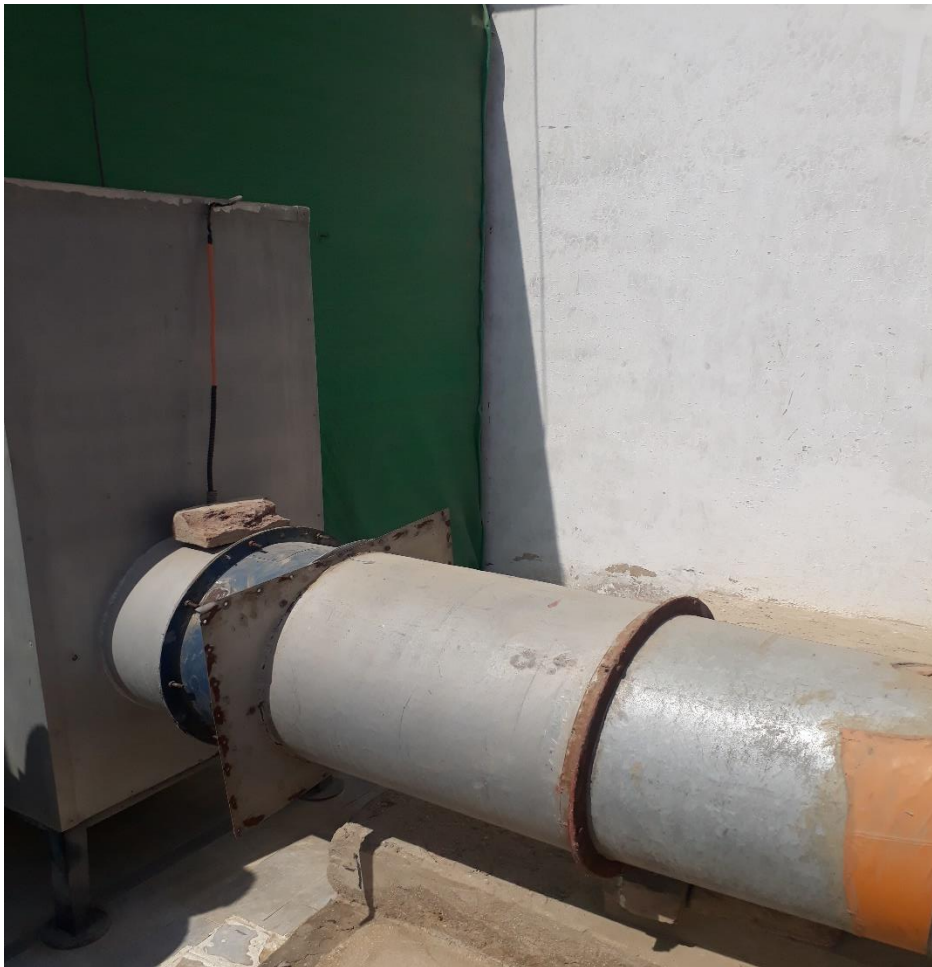
Figure 10: A duct for solar drying unit
